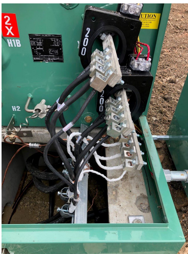
Figure 13 – A single-phase transformer with current transformers (CTs) mounted on the low-voltage bushing terminals and a customer-supplied cable management system at the entrance to the precast vault
